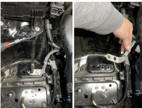
10. Using a 12mm socket, loosen and remove bolts to disconnect the chassis ground. Save bolts for use later.
